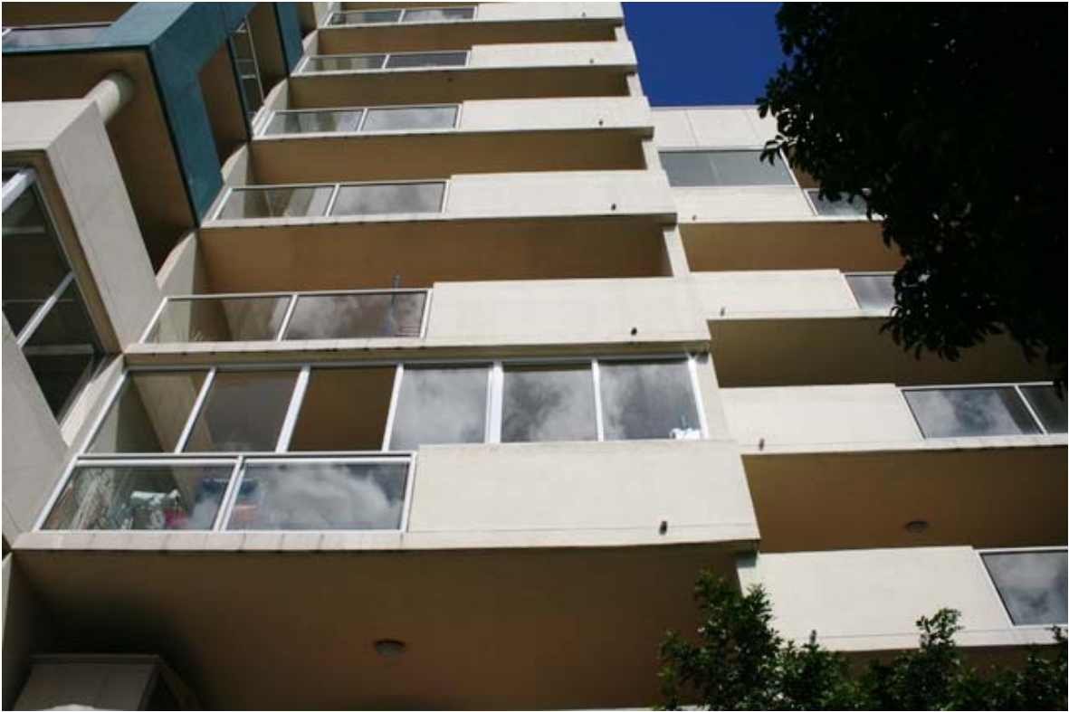
Photo 11– Sliding windows to balcony with a solid and glazed balustrade from the street.
