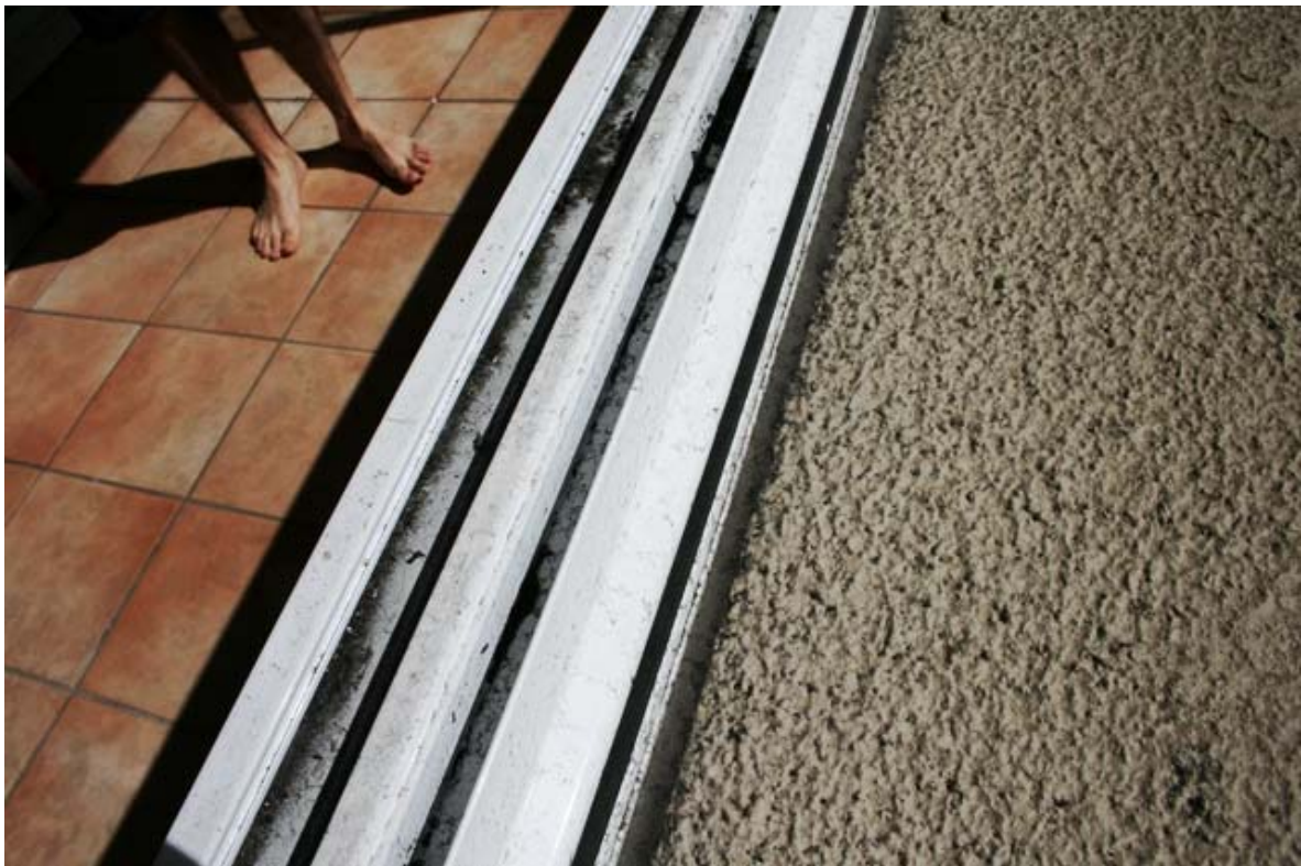
Photo 2 – Sliding window sill track fixed to the inside face of the solid balustrade.
