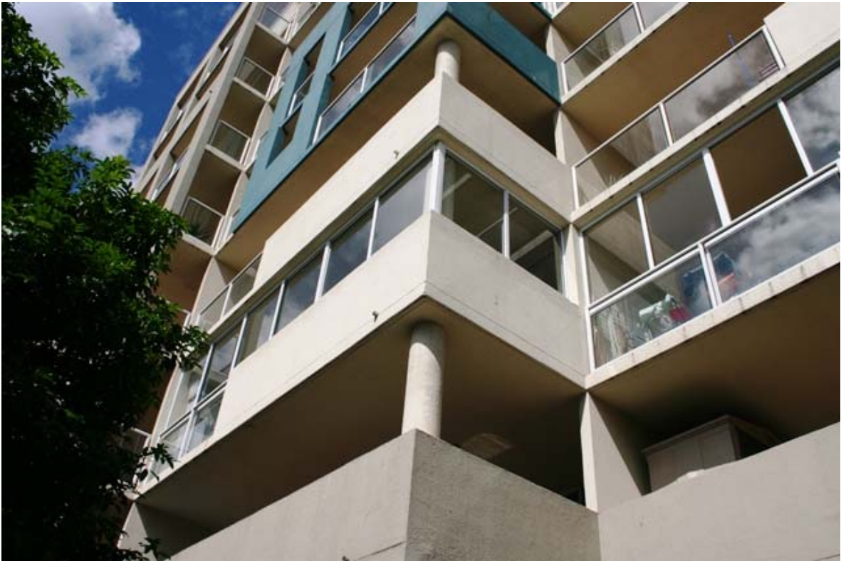
Photo 12 – Sliding windows to balcony with a solid and glazed balustrade from the street.
