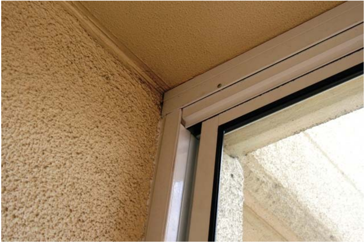
Photo 3 – Sliding window head track and jamb, fixed to soffit and rendered masonry wall.
